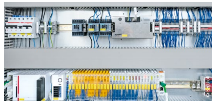
Complete control and monitoring of the prototype runs on a CX2040 Embedded PC (bottom left) with Intel® Core™ i7 CPU and four processor cores.
