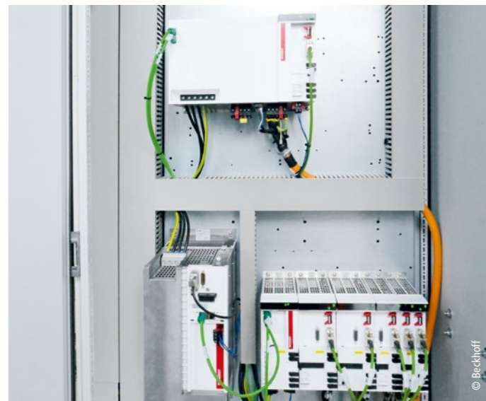
The AX8000 multi-axis servo system, in combination with the AX5000 Servo Drive (bottom left), controls the high-performance spindle and the servo drives installed in the axes of the CNC robot.
