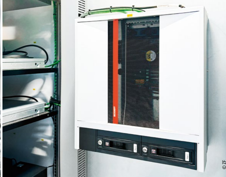
The high-performance C6675 control cabinet Industrial PC forms the core of the control system for the new ZF production line.
