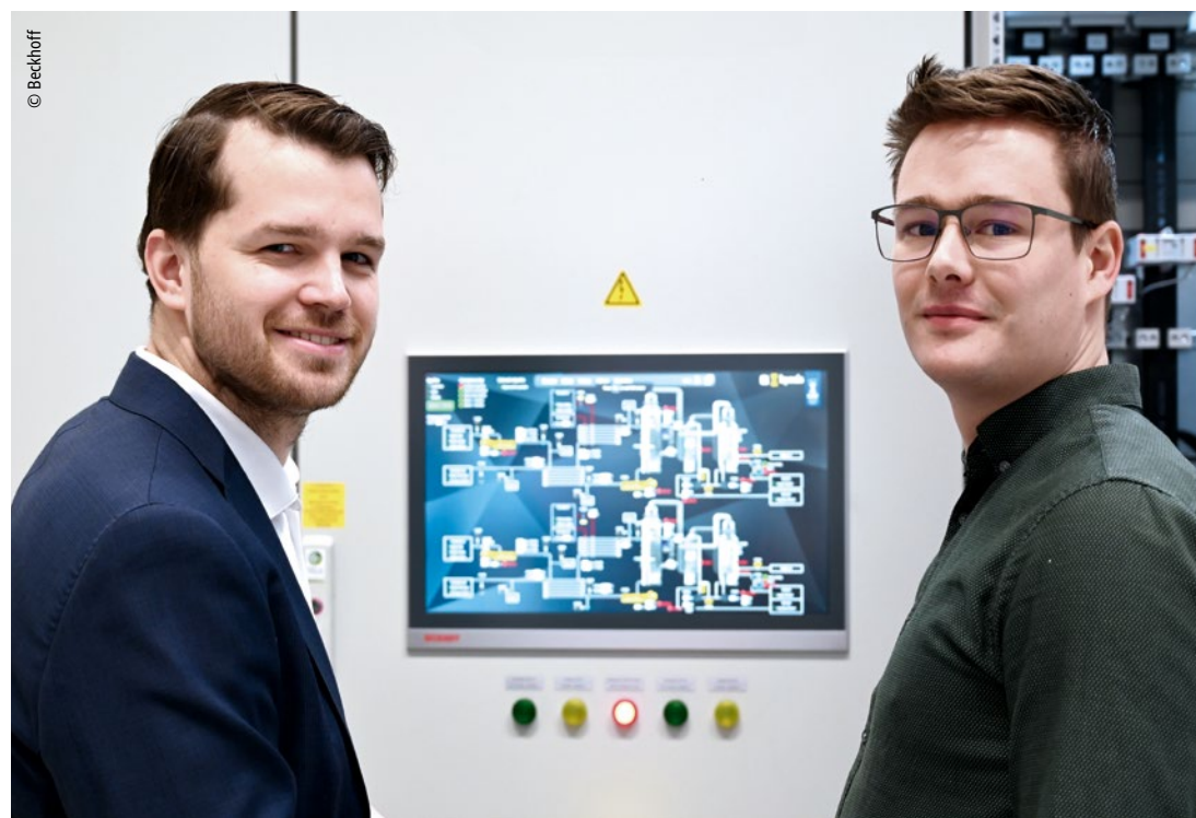
Reinoud van Bennekum (sales engineer at Beckhoff Netherlands – left) and Dylan Veelers (project engineer at Byosis – right) pictured with the central control cabinet with a CP2921 multi-touch Control panel
