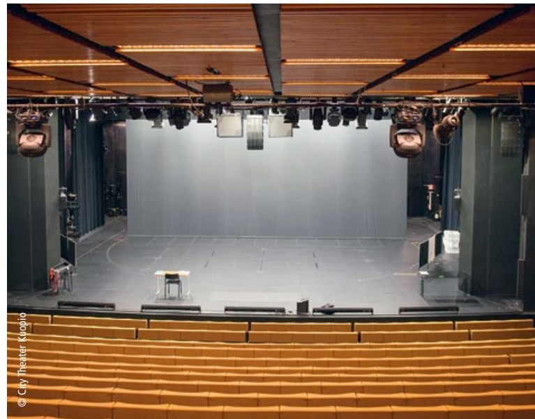
Based on a PC- and EtherCAT-based control platform, the City Theater in Kuopio accommodates flexible and independent control of the DMX environments, integrated light switches and buttons, and the ability to integrate third-party systems.
