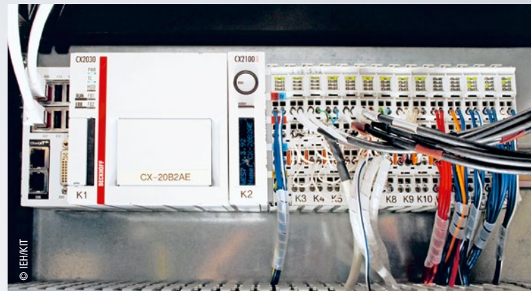
For inverter emulation, the CX2030 Embedded PC enables short control cycle times of 50 \mu s.
